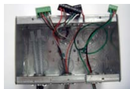
Single gang electrical box housing the RPS
